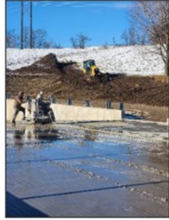
Figure 3. The contractor works on cutting grooves in the floor for hoof traction.
