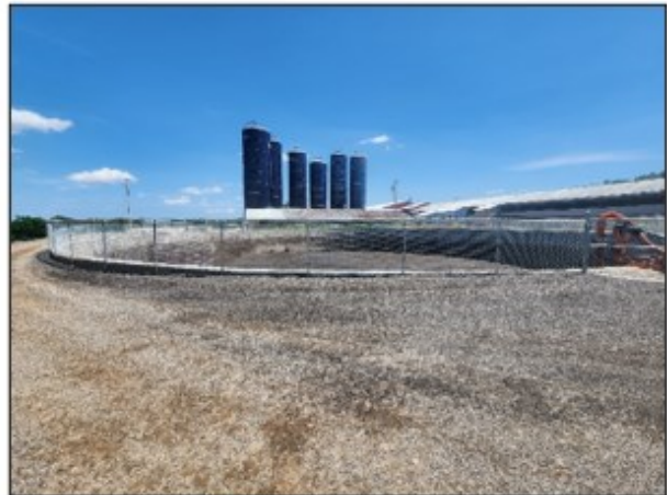
Figure 4. The manure storage with safety fencing, signs, and gates.
