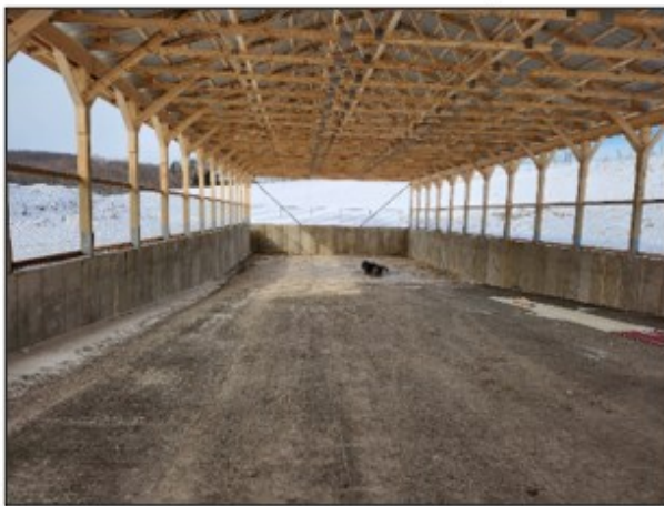
Figure 4. The newly constructed covered waste storage eliminates potential runoff from manure piles.
