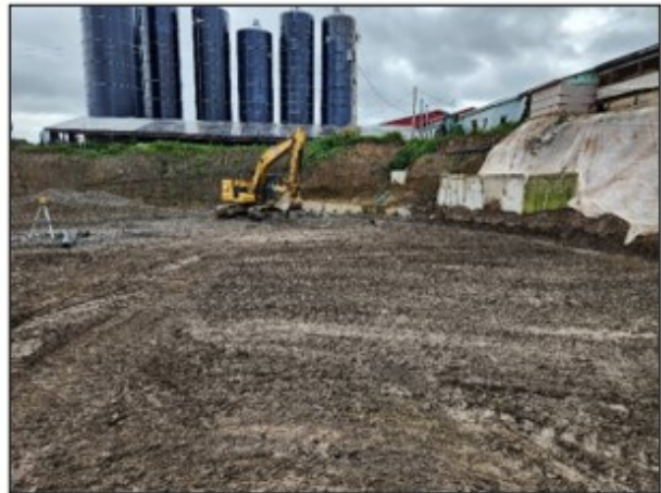
Figure 2. The contractor works on a solution to keep the soil from sloughing.
